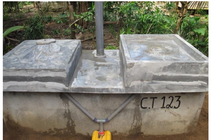
The kind of sanitary latrine installed in the urban commune of Maroantsetra: EcoSan latrine.
